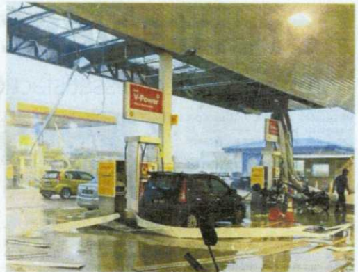
Extensive damage: Debris lying in between petrol pumps and vehicles at a Shell kiosk in Sungai Besi.
