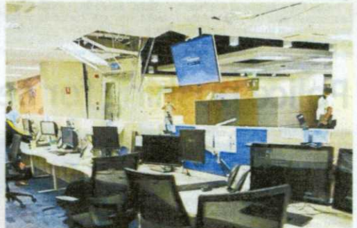
Office mess: Staff of the Standard Chartered Bank branch at Wisma Scope International, next to Kuala Lumpur-Sungai Besi Highway, viewing the damage to the ceiling after the storm.
